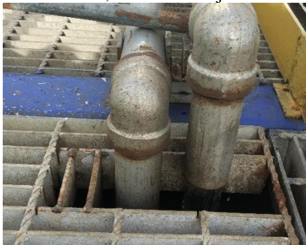
Gambar 7. Pipa Output Pompa
